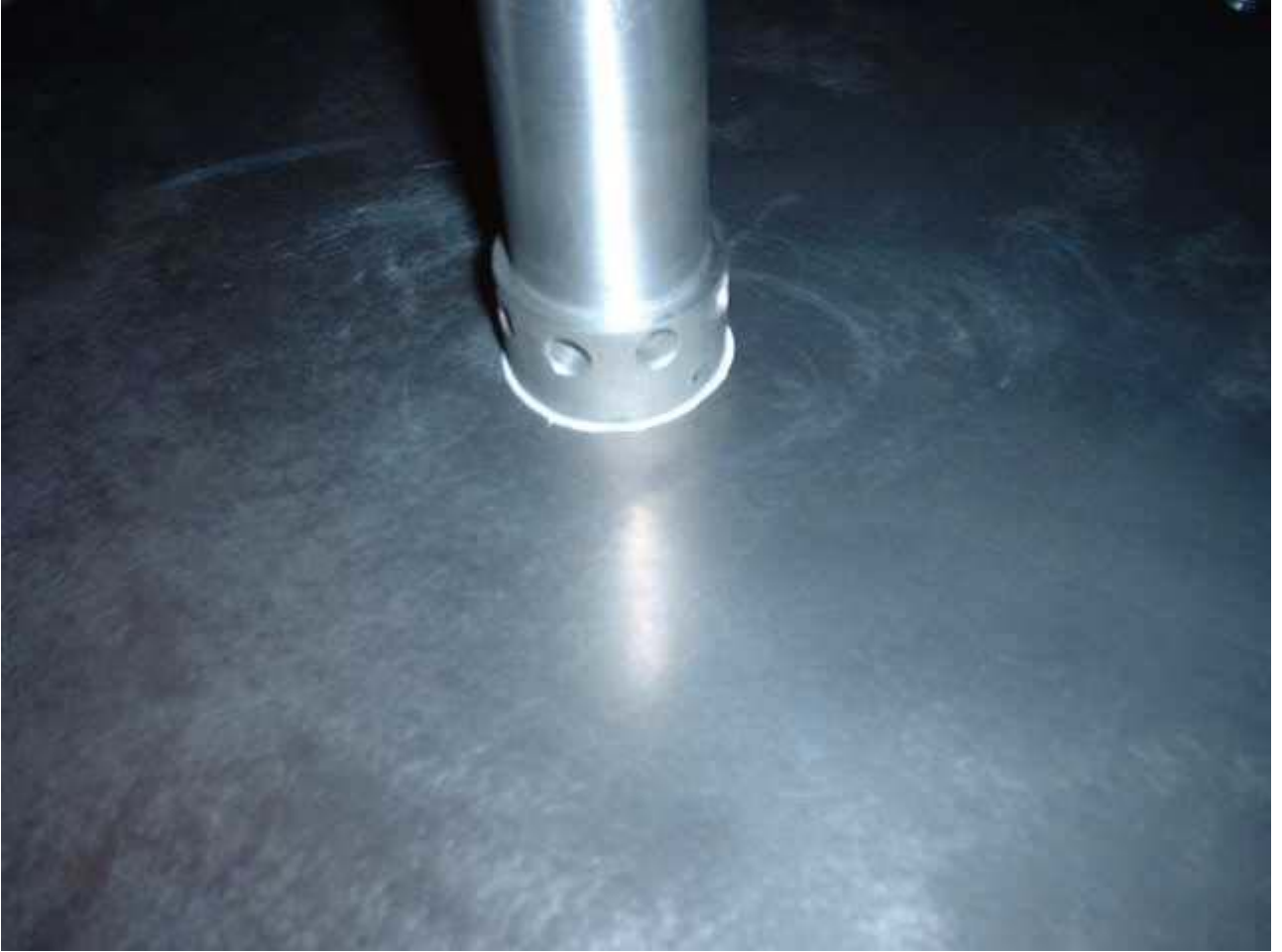
Heat exchanger assembled and ready
